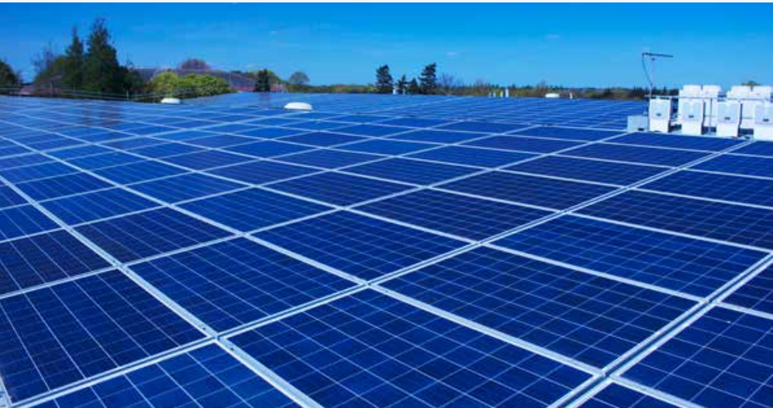
360kW solar panel installation on the roof of the Newmarket Road store in Bury St Edmunds.
