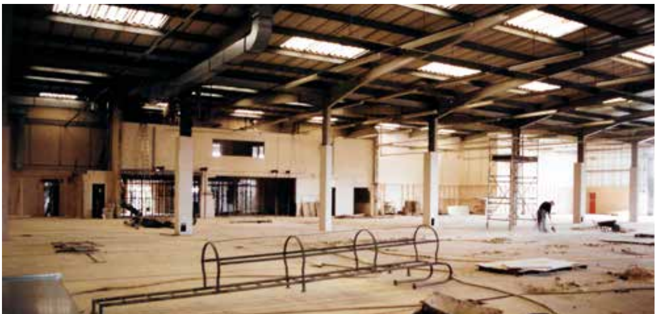
Under construction, the World of Furniture store was refurbished in just 10 weeks.
